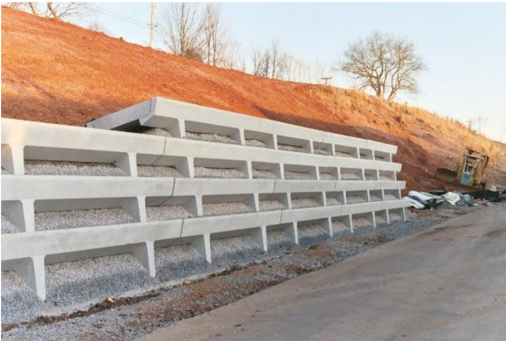
After the units are in place, TANG chose to fill the units with stone. Another option was to plant the front of the units as seen in the picture below.
